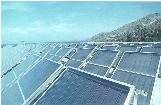
Fig. 1 Solar collectors mounted on a flat roof.
